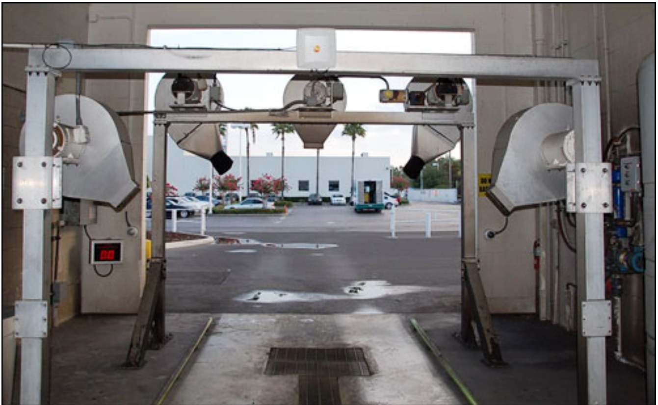
An RFID reader and antenna were also installed at Fields BMW Winter Park's car wash.
